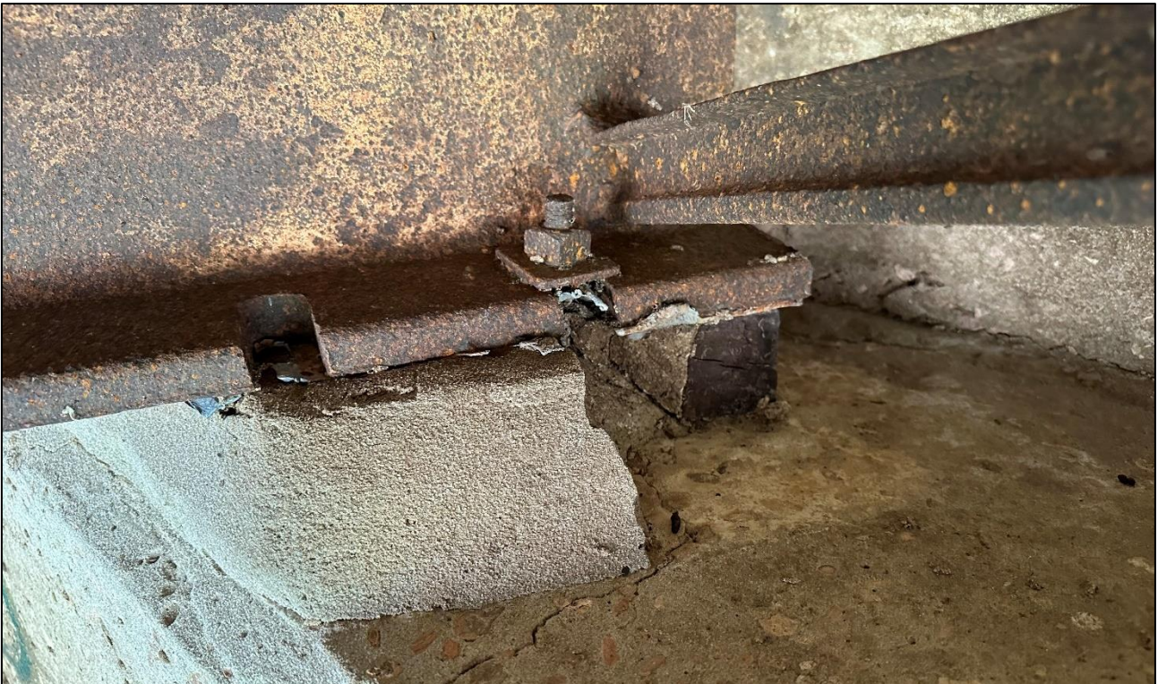
Photo 4 - Fragments of grout beneath an end bearing had been washed away by floodwater
