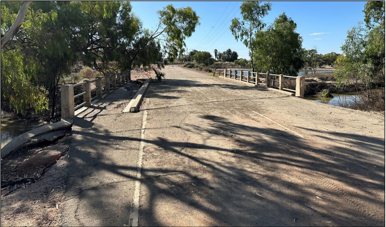
Photo 1 - Cracking and subsidence to road surface at the bridge approach
