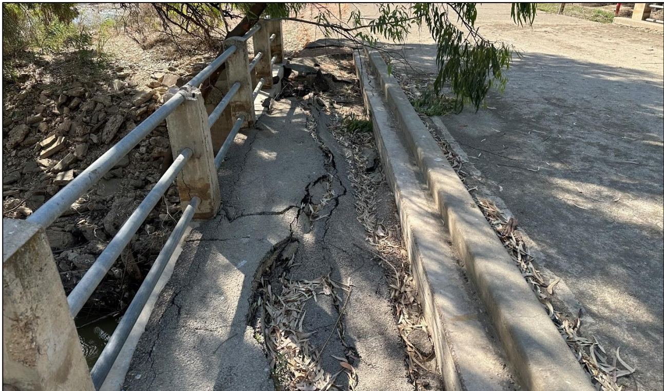
Photo 3 – Severe deterioration & erosion of pedestrian footpath
