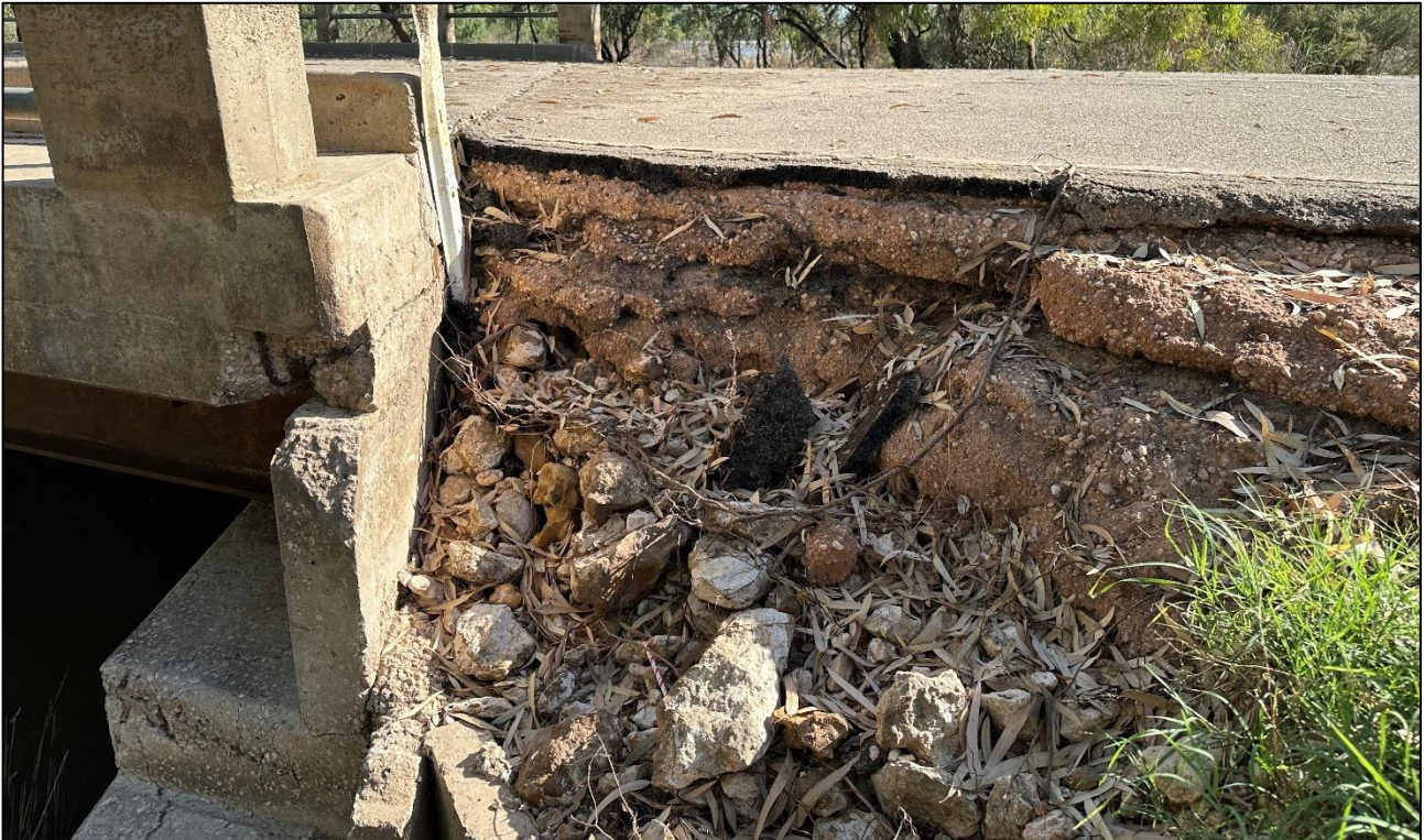
Photo 2 - Erosion of road layers
