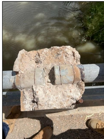
Photo 19 – Deterioration of concrete post exposing corroded reinforcement
