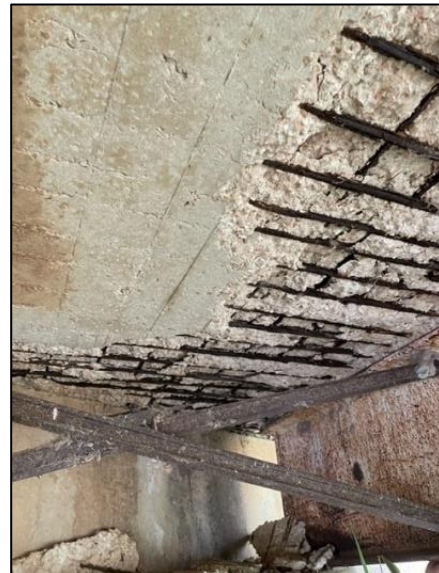
Photo 9 – Concrete delamination and spalling from bridge soffit on west end.
