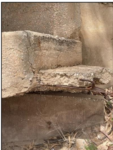
Photo 4 – Concrete degradation showing exposed reinforcement of concrete support beam on East end of bridge.
