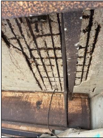
Photo 6 – Concrete delamination and spalling from bridge soffit on east end.
