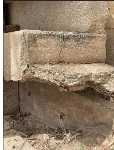
Photo 3 – Concrete degradation showing exposed reinforcement of concrete support beam on East end of bridge.
