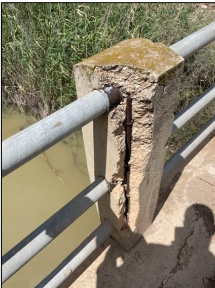
Photo 18 – Deterioration of concrete post exposing corroded reinforcement
