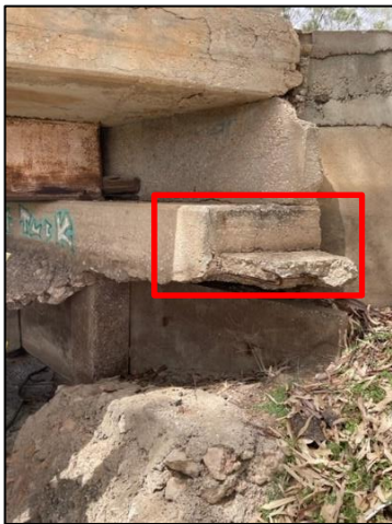
Photo 2 – Concrete degradation showing exposed reinforcement of concrete support beam on East end of bridge.
