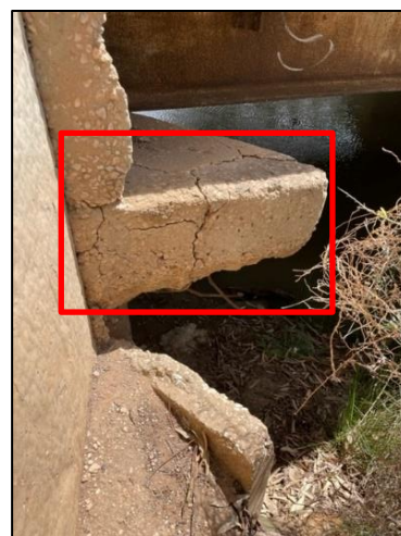
Photo 5 – Concrete degradation showing exposed reinforcement of concrete support beam on East end of bridge.
