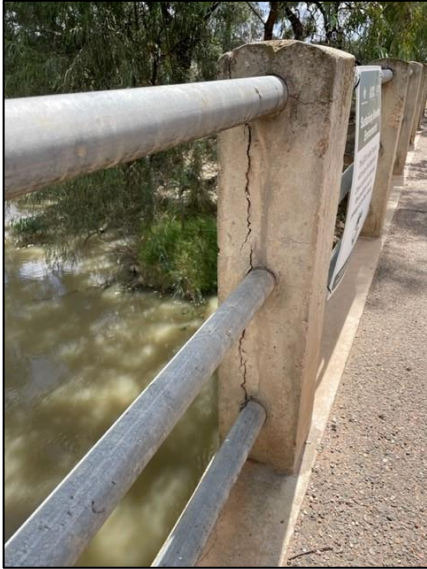
Photo 16 – Cracked Concrete post of hand rail system.
