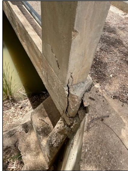
Photo 17 – Evidence of impact damage to concrete post.
