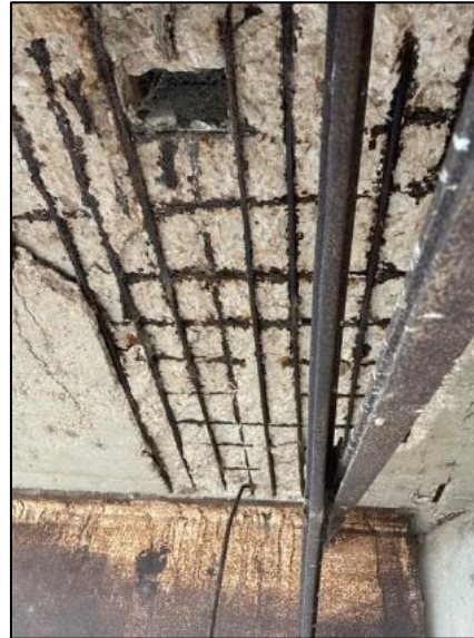
Photo 7 – Concrete delamination and spalling from bridge soffit on east end.
