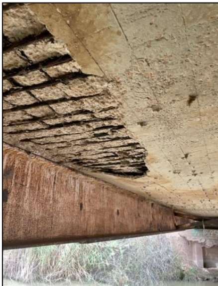
Photo 8– Concrete delamination and spalling from bridge soffit on west end.
