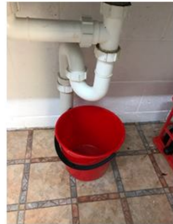
Bucket used for the leaks from the sink
